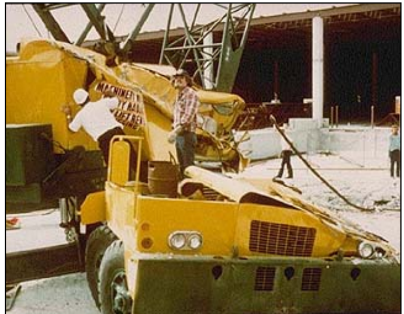
Crane accidents cause damage, injury and death.
