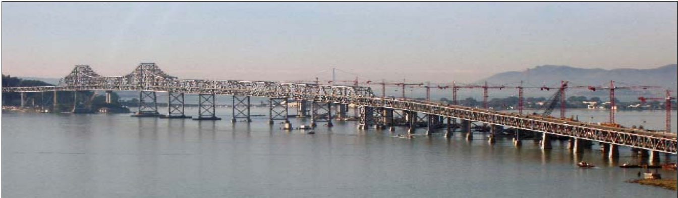
California is the most recent state to enforce crane operator certification requirements. Shown here is the San Francisco Bay Bridge project, one of thousands of jobs in the state employing the use of cranes.
